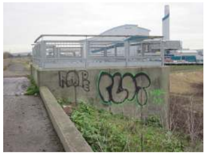
Some of the graffiti issues we've been experiencing
