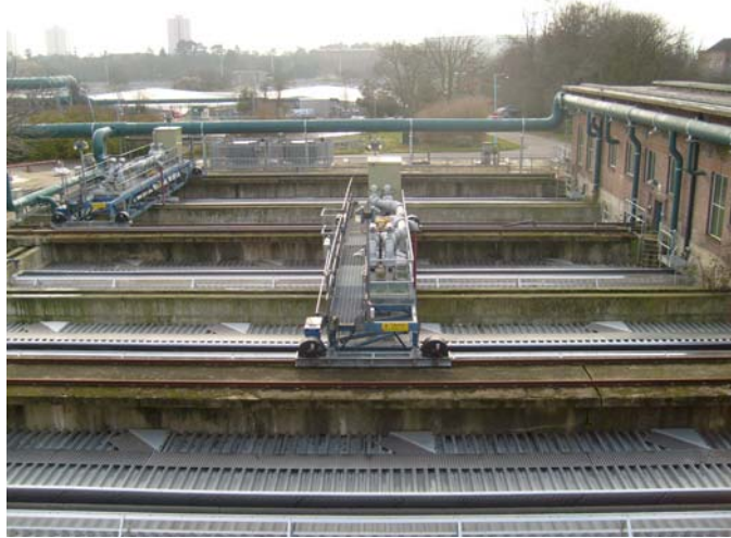
CV Grit Channels and Dredgers (East)
