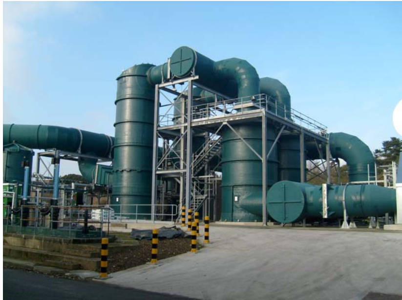
Odour Control Unit (East)
