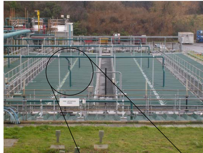
Pre-Aeration Lanes (West)
