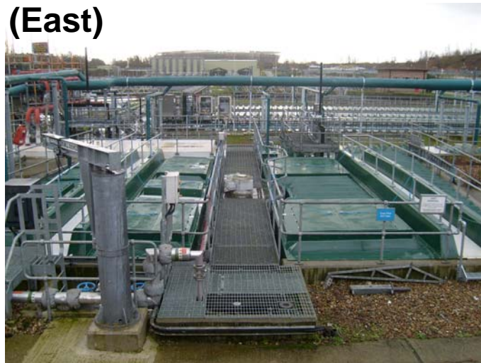
Cross Flow Grit Traps (West) Thames Water
