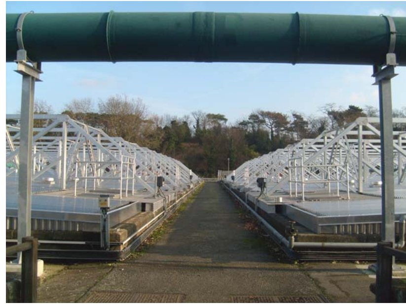
Storm Tanks 4 & 5 (East)
