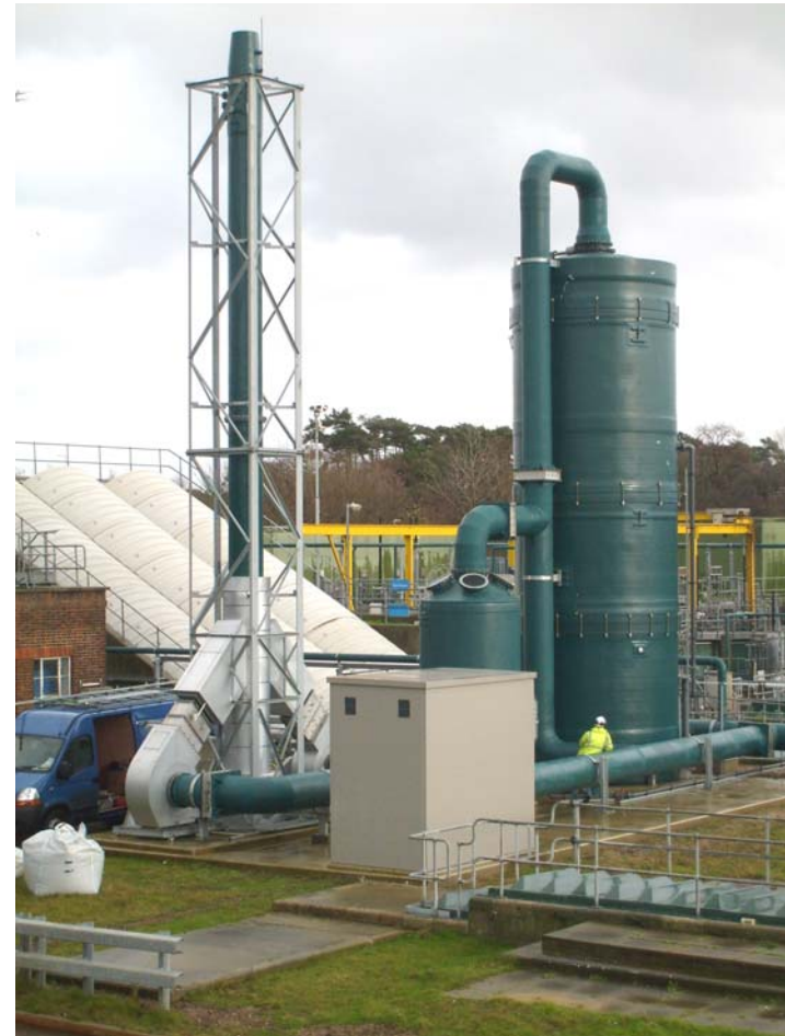
Odour Control Unit (West)
