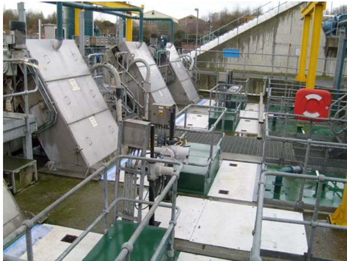
Fine Screens (West)
