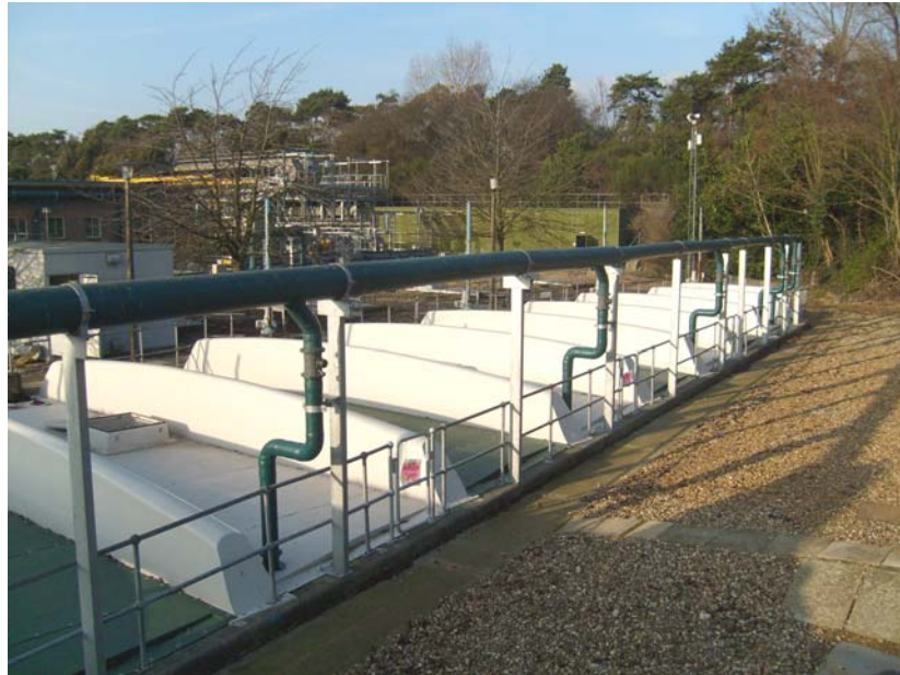
Storm Weir (East)
