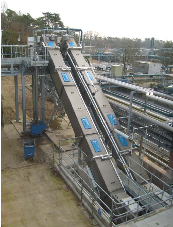
Screen Conveyors (East)
