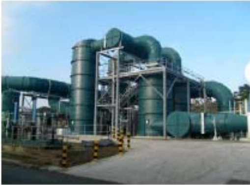
Odour Control Unit (East)
