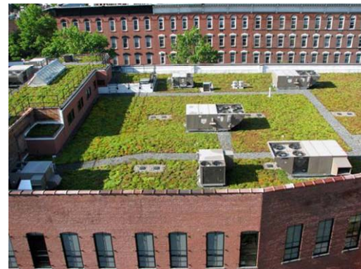
Green roofs to attenuate and absorb rainfall
