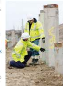
Assistant Engineer James Clark (left) inspects the piling with a representative from Black & Veatch.
