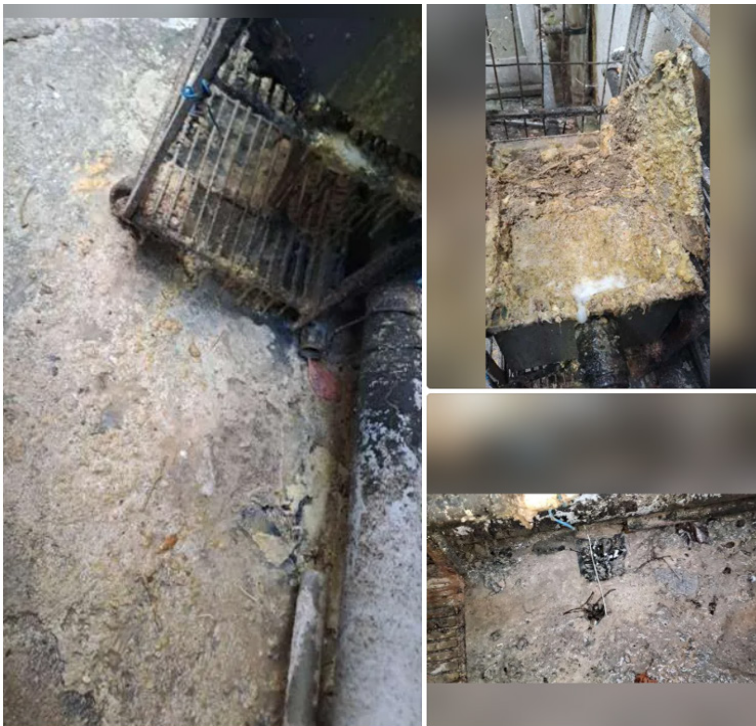
Fat, oils and grease poured into a sewer by a takeaway
