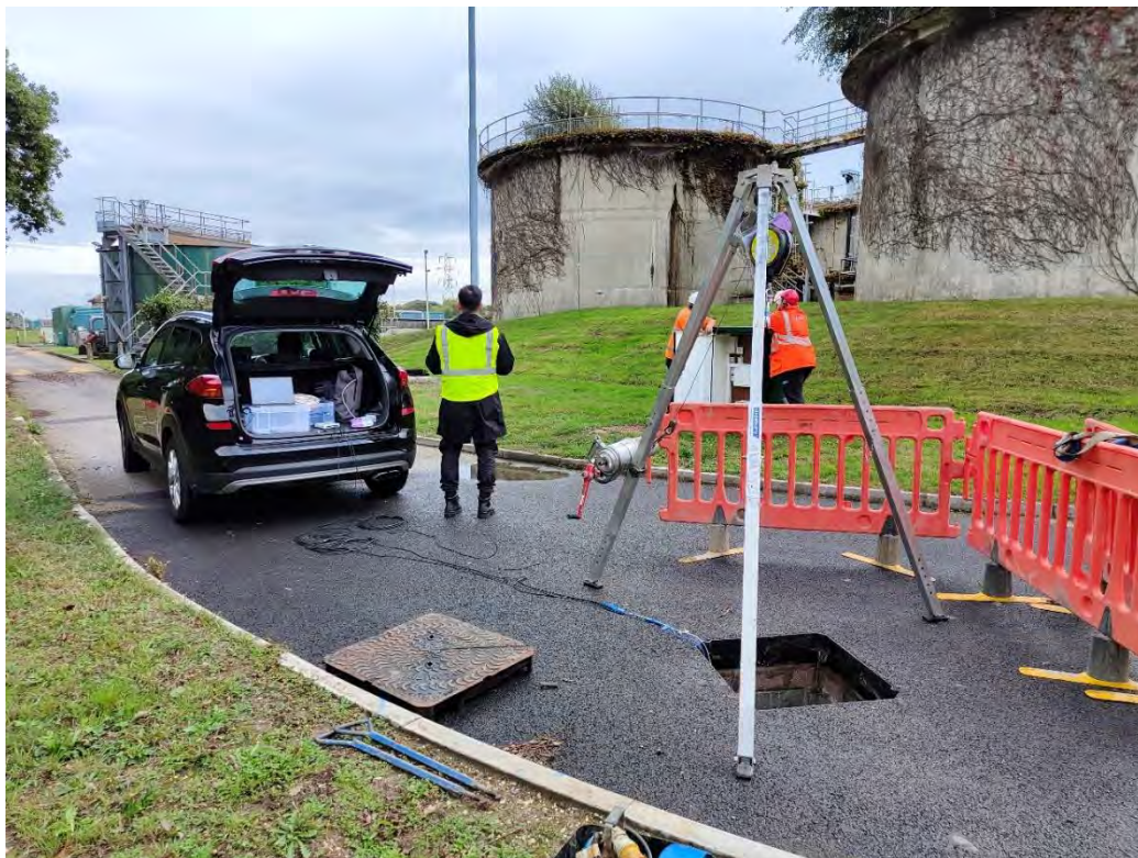
Data acquisition equipment on site
