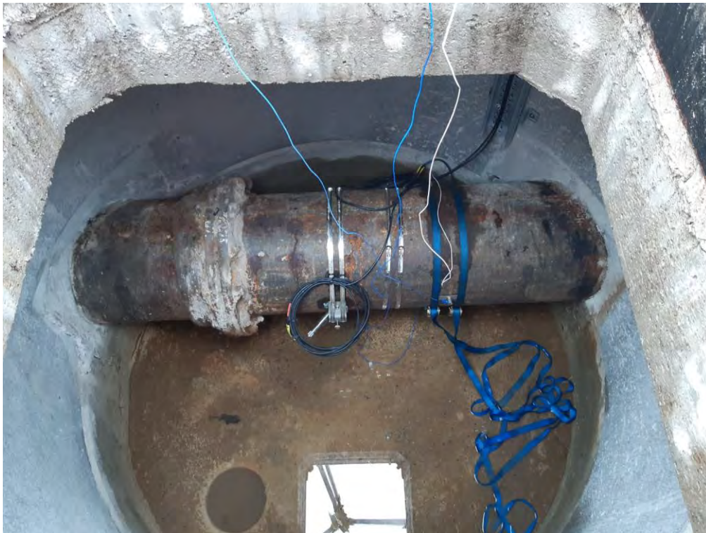
Accelerometers attached to the pipe
