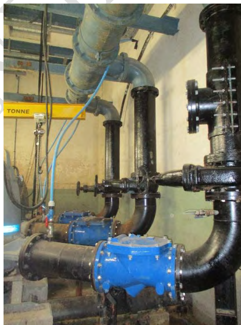
Figure 9 – 3 pumps in underground dry well
