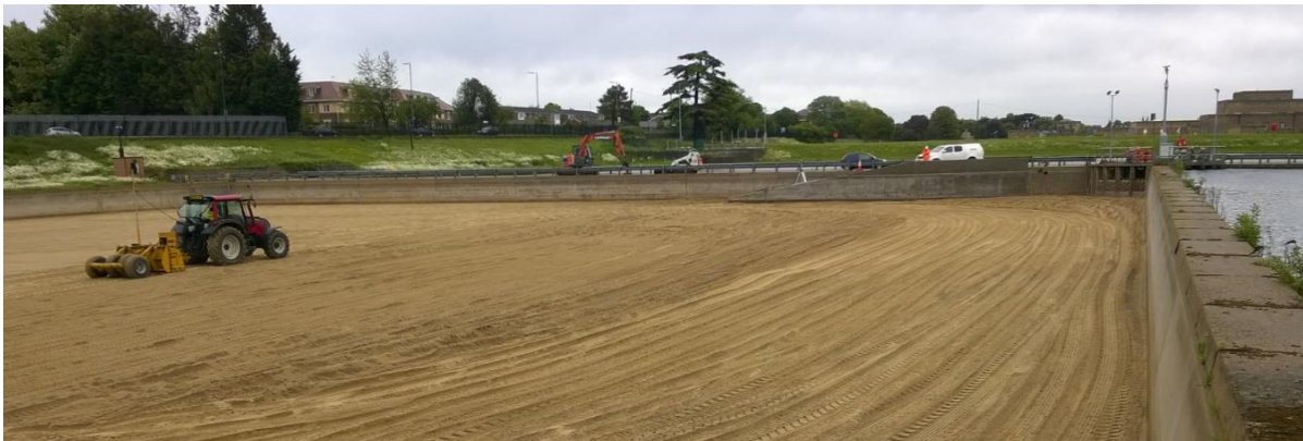
Figure 3.9: An example of a large slow sand filter in London (Hampton WTW) being rebuilt following porous floor maintenance and one adjacent filter in service (RHS of photo)
