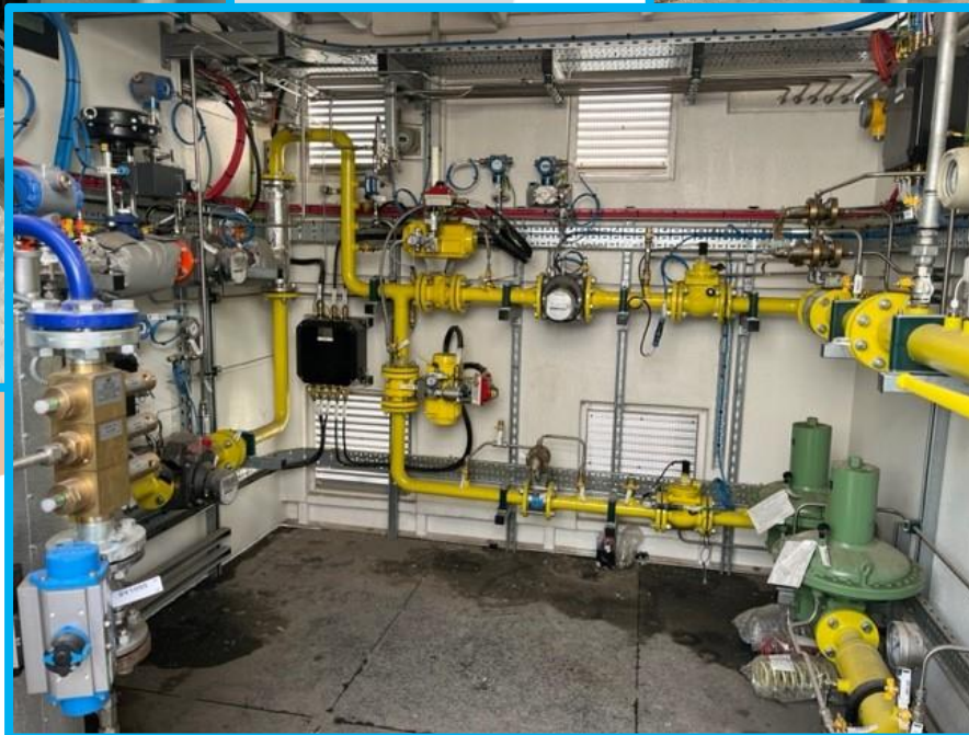
Main Gas-to-Grid propane dosing valves, export valve and PRVs
