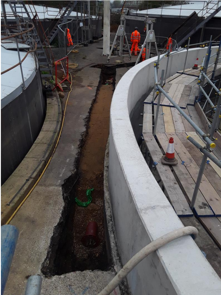
Digested sludge pipeline
