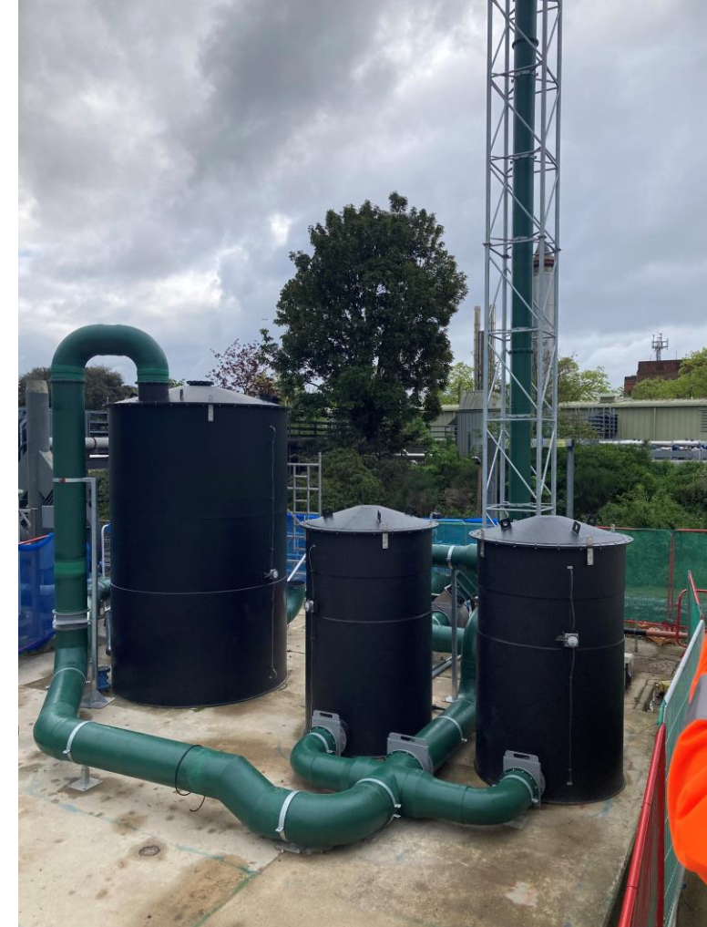
Sludge Area - New OCU
