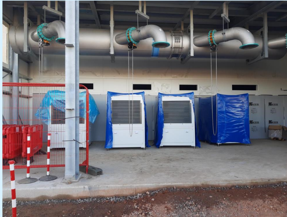
New LV Blowers
