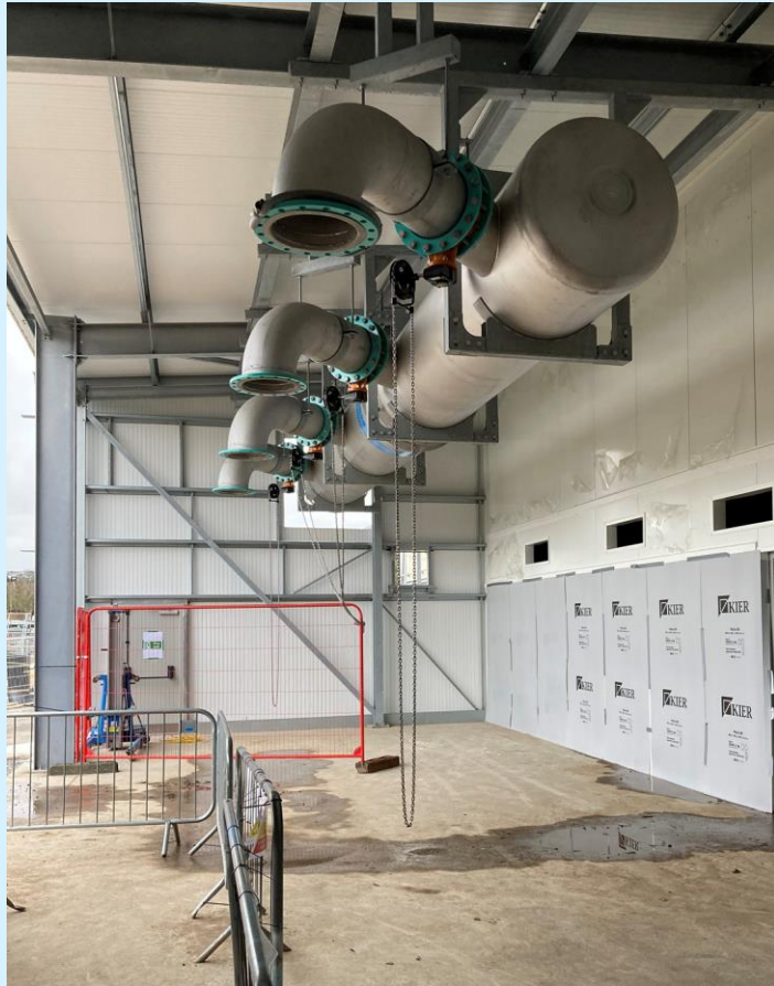
Blower building air header
