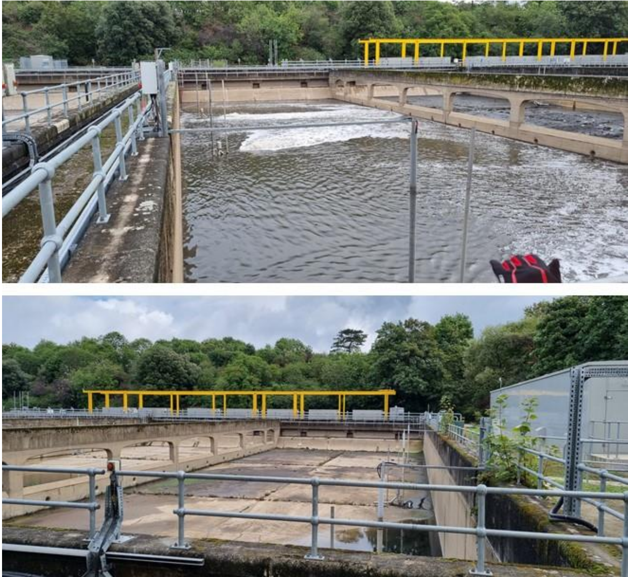
Figure 4: Existing Mogden STW storm overflow tanks, on top of which the TTP will be constructed
