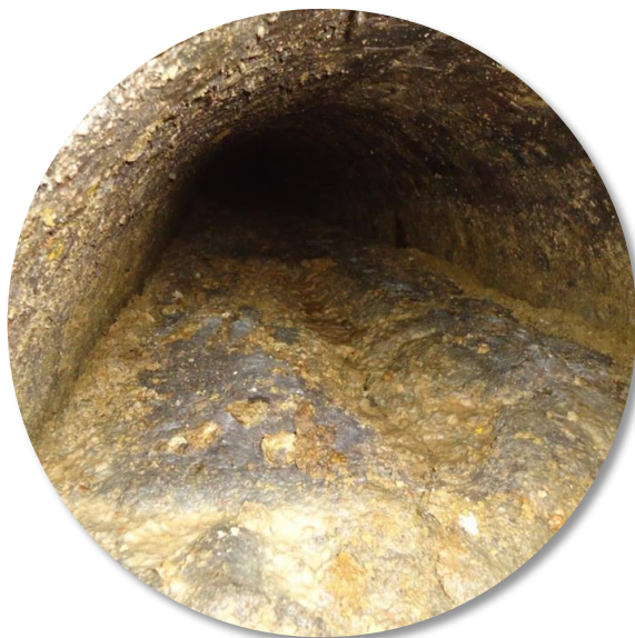
FOG builds up over time so that it can partly or totally obstruct our sewer pipes, lead to flooding of properties.
